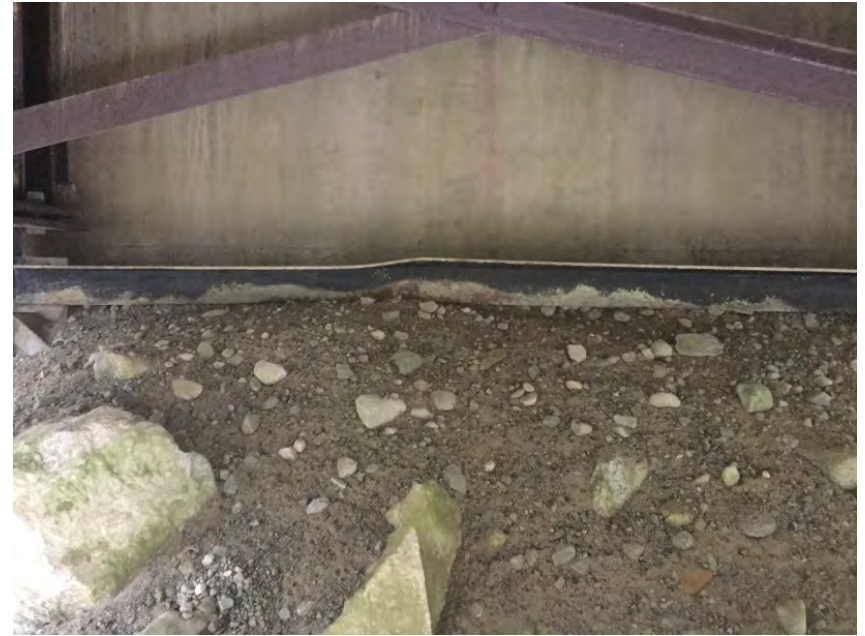
Minor damage to right bank bracing
