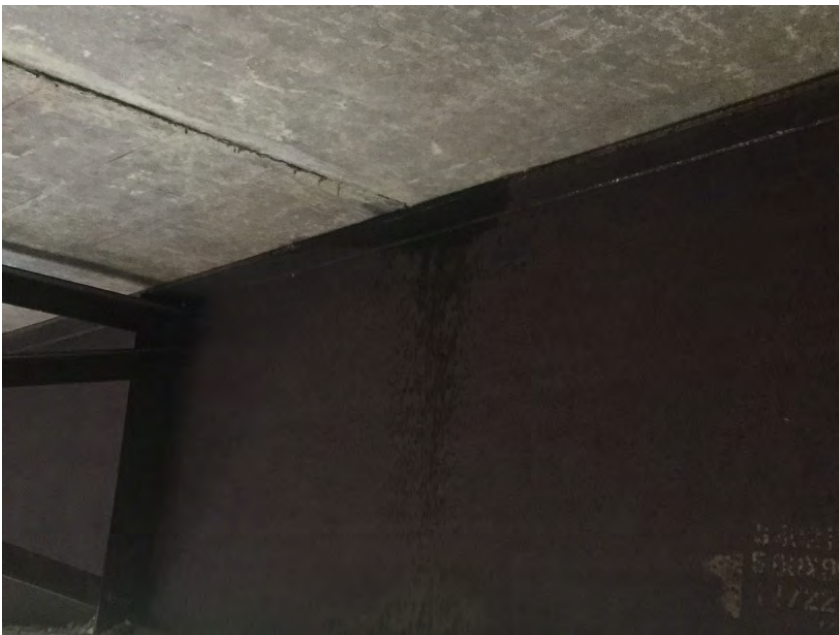
Evidence of water getting through random deck joints
